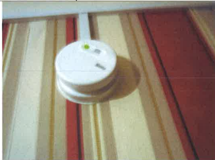
Smoke alarm in hall
