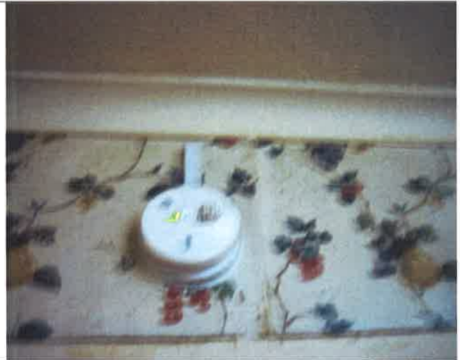
Heat alarm in Kitchen
