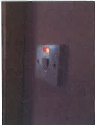
Hall - kitchen light switch
