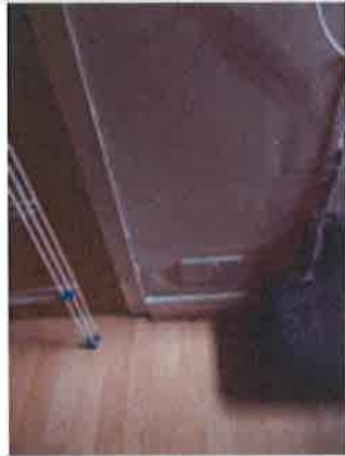
Hall - double socket - disconnected
