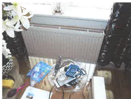
3. New radiator living room
