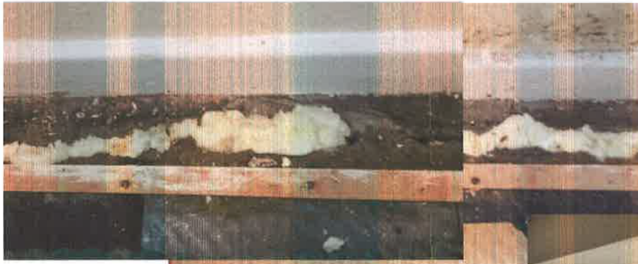
2a) As at 9/10/15 2b) As at 26/04/16 showing mildew (probably due to condensation)
