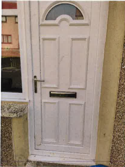
Damaged and insecure front door - March 2017
