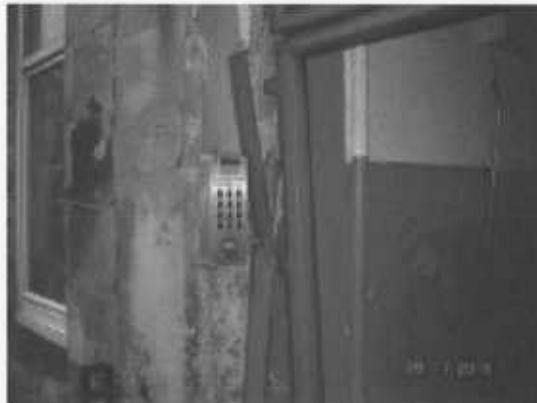
VANDALISED DOOR ENTRY
