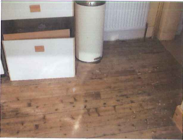
4: Missing kitchen floor covering
