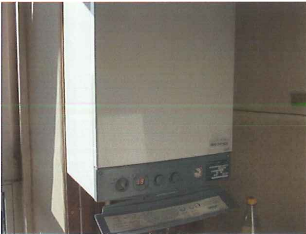
8: Central heating boiler
