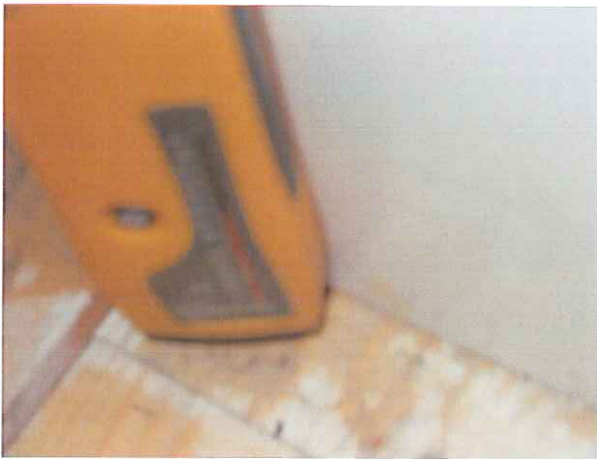
2: Damp meter/dry damp stain bathroom floor
