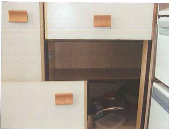
6: Defective kitchen units
