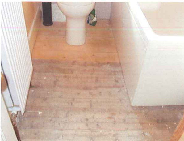
3: Missing bathroom floor covering
