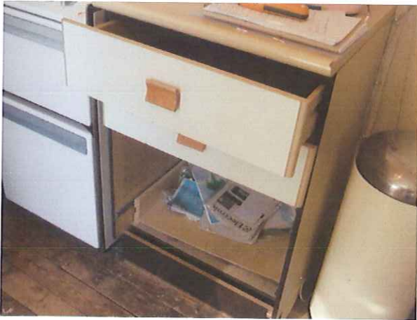
5: Defective kitchen units
