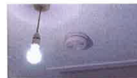
(Ph17) Hall cupboard – Smoke detector
