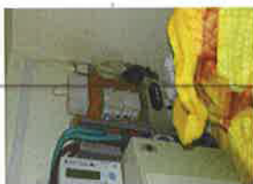
(Ph15) Hall cupboard - switchgear
