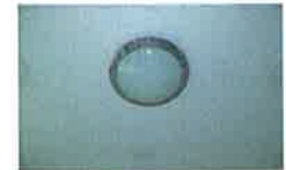
(Ph18) Bathroom – Ceiling light
