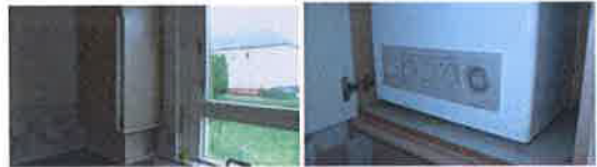
(Ph5) Kitchen – Boiler cupboard (Ph6) Kitchen – Boiler
