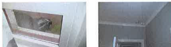
(Ph13) Lounge – Misting in sealed unit (Ph14) Lounge – Smoke detector
