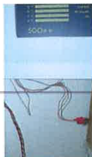
(Ph16) Hall cupboard – Alarm box
