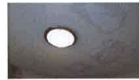
(Ph9) Kitchen – Ceiling light
