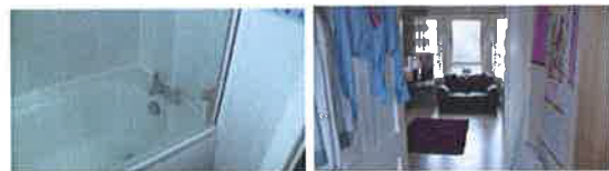
(Ph11) Defective R/H bath tap (Ph12) Lounge – From Kitchen
