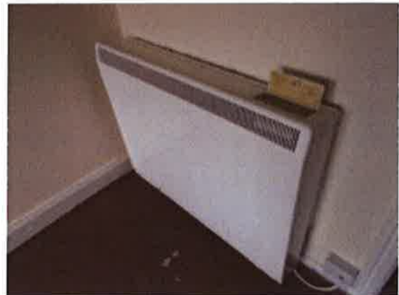
Bedroom (1) - Night storage heater
