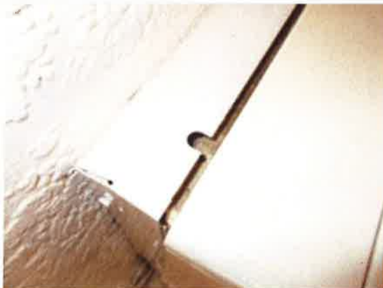
Hall - Night storage heater - unsecured to wall fixture/gap
