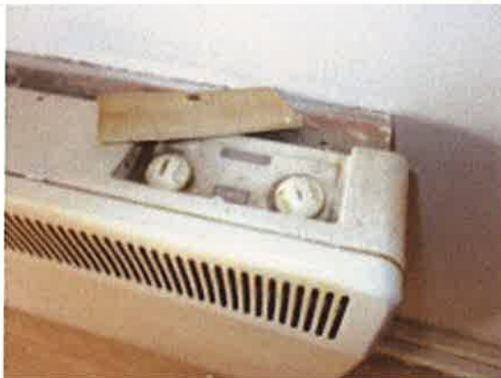
Living Room - Night storage heater - loose/ broken cover to controls
