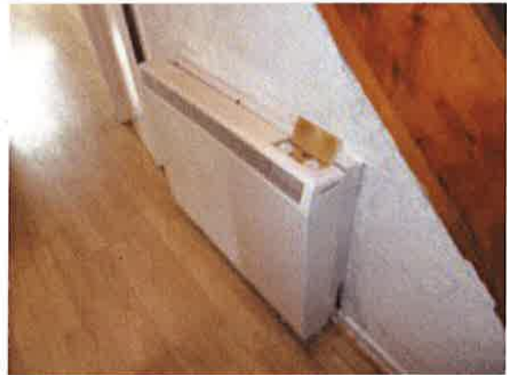
Hall - Night storage heater
