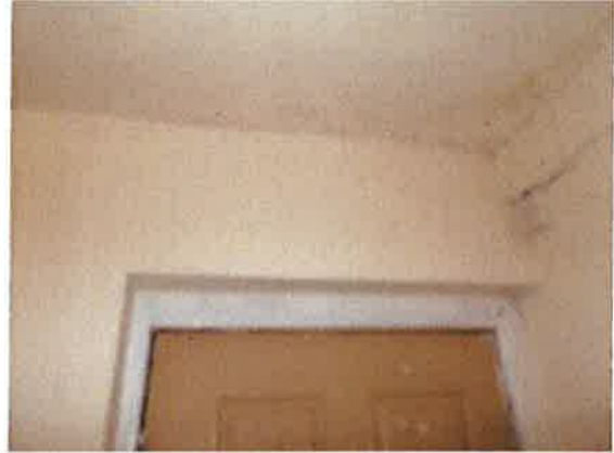
Hall - walls above front door - slight water stain to ceiling in corner.
