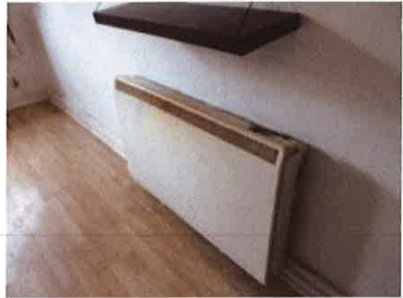
Living Room - Night storage heater
