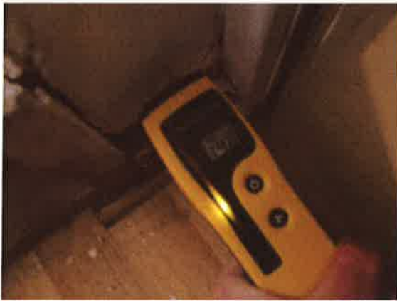
Hall - left side of front door - moderate damp reading to base of wall
