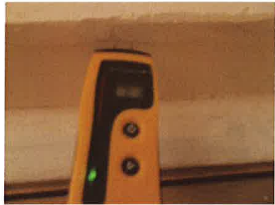
Hall - lintel above front door - low damp reading
