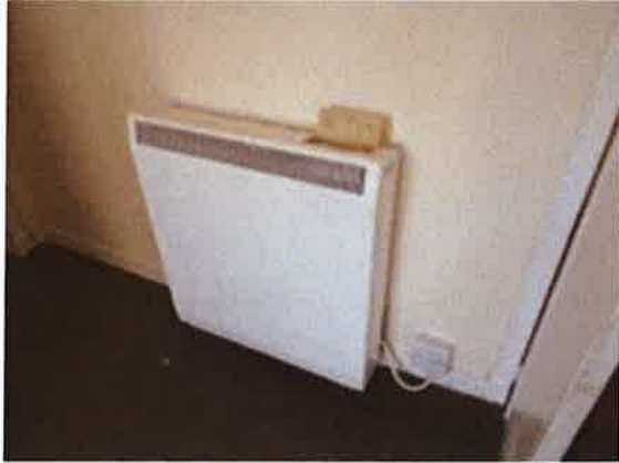
Bedroom (2) - Night storage heater
