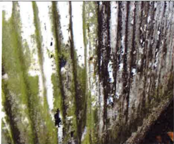
Photo 3 – Further holes/rust in cladding
