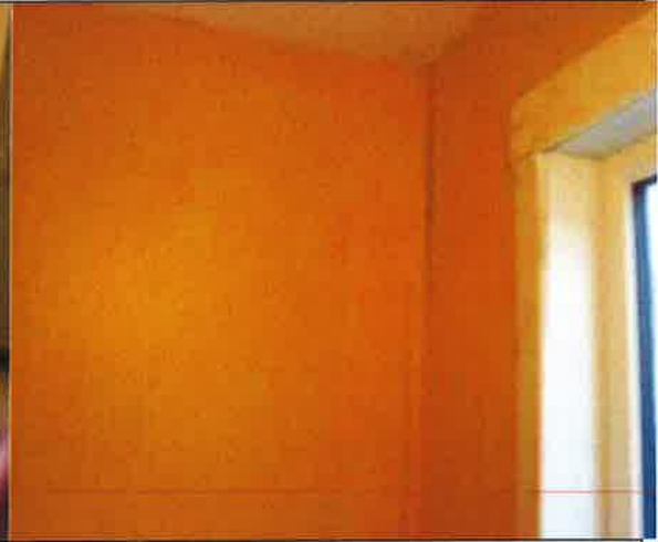
Photo 14 – Loose tape bathroom
