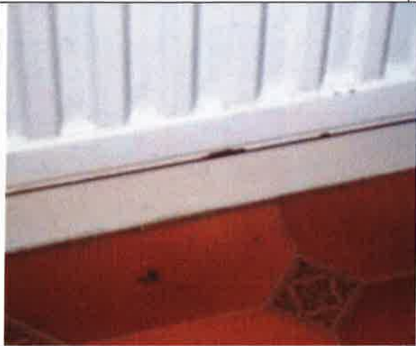
Photo 11 – Rust on radiator
