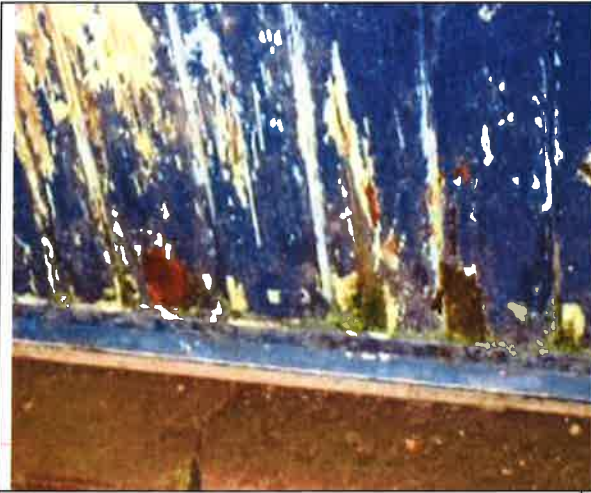
Photo 9 – Rotted rear door
