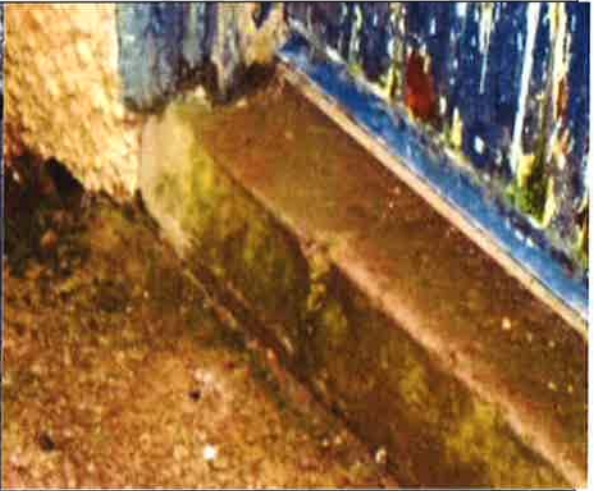
Photo 8 – Broken rear step
