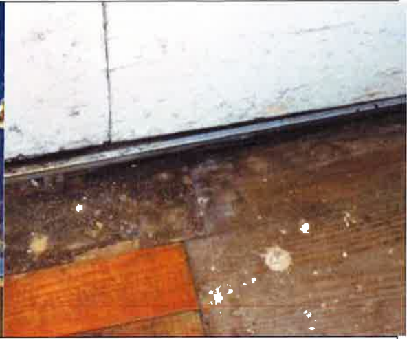
Photo 10 – Rotted floor rear door
