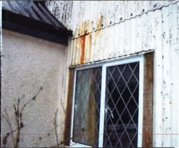
Photo 2 – Holes/rust cast iron cladding
