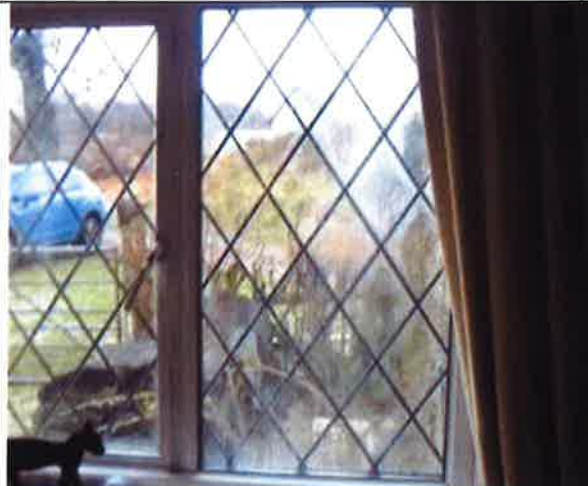
Photo 15 – Defective double glazed unit
