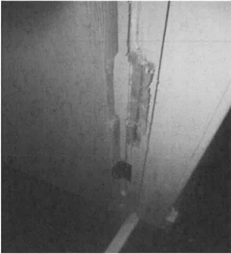
Ill-fitting bedroom door
