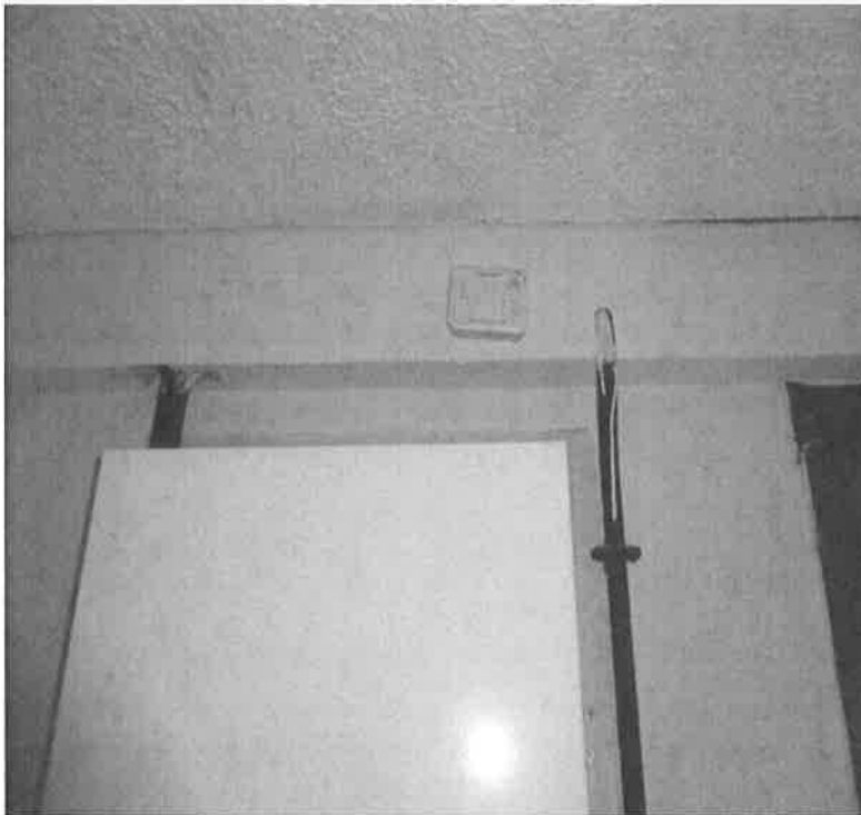
Kitchen – Carbon Monoxide detector
