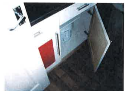
06 - Kitchen, faulty cupboard units
