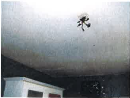
04 - Kitchen, missing light
