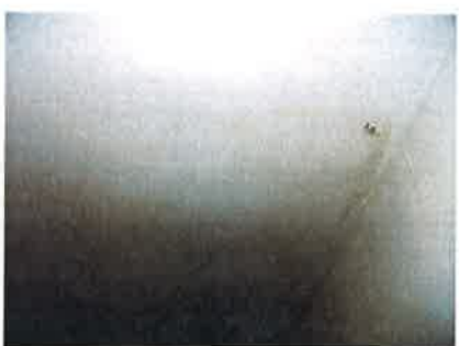
09 - Bedroom, damp stain on ceiling
