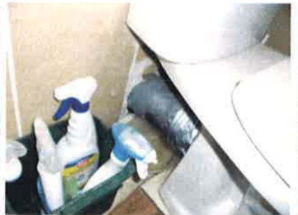
08 - Bathroom, leak at WC
