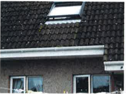
07 - Rear gutters with vegetation
