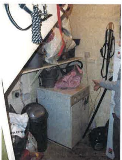
12 - Oil fired boiler (no CO detector) (last serviced at tenant's expense)
