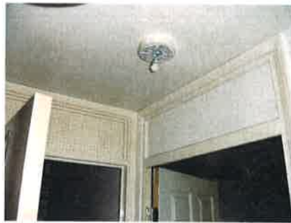
02 - Lower hall, missing smoke alarm
