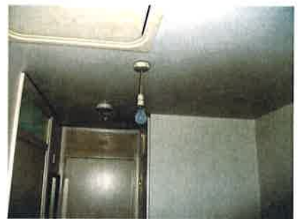
03 - Upper hall, missing smoke alarm
