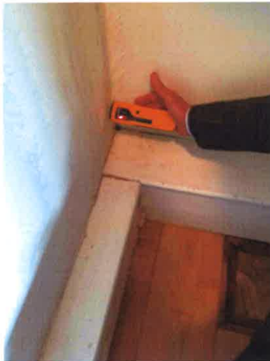
Dampness below boiler
