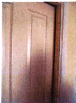
11. Badly fitting cupboard door
