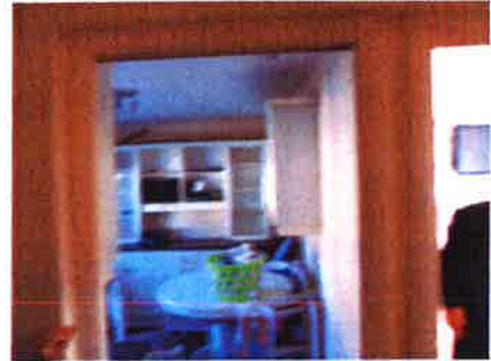
10. Missing kitchen door
