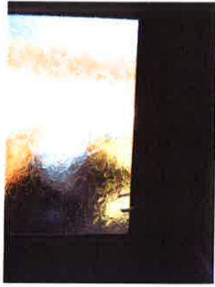
14. Front entrance door
