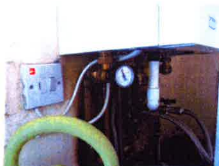
3. Pressure gauge and piping at boiler
