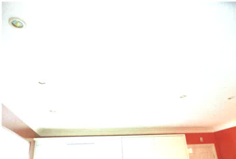
Kitchen light fittings. None in working order
