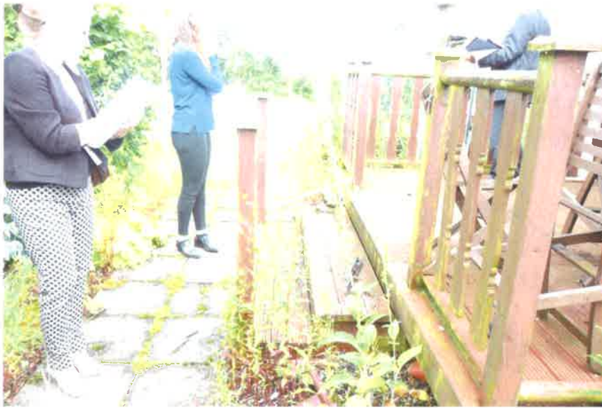
Patio steps. Fence and handrail to each side missing
