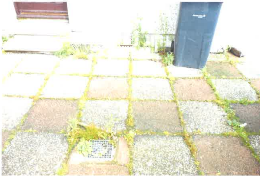
Yard and kitchen drain.
