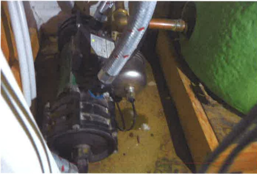
Shower pump. Note leakage from pump which runs under laminate floor
