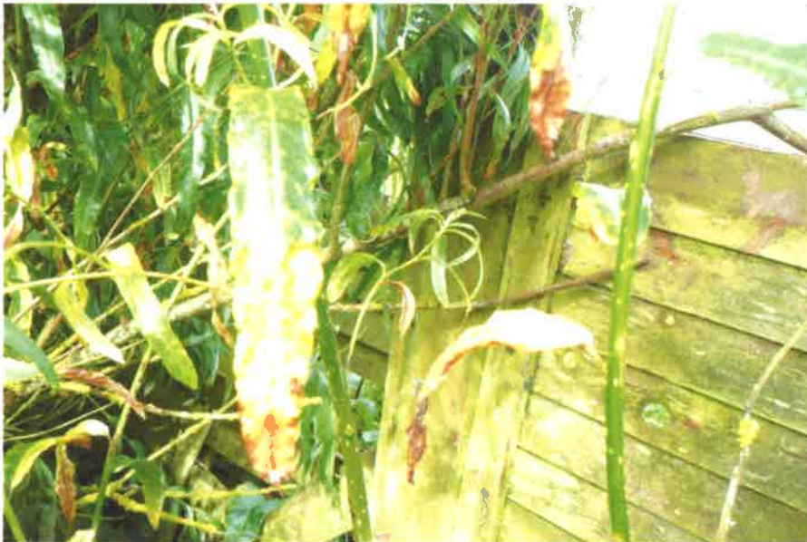
Garden fence. Panel damaged to rear of tree.
