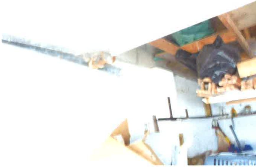
Garage door – left hand stop end to track missing
