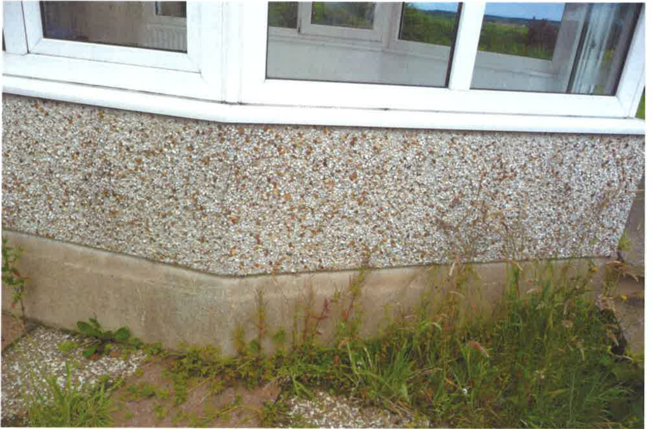
Cracked harling at corner and to courses in plaster below.
