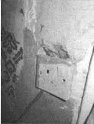
Socket in back room - exposed wiring
