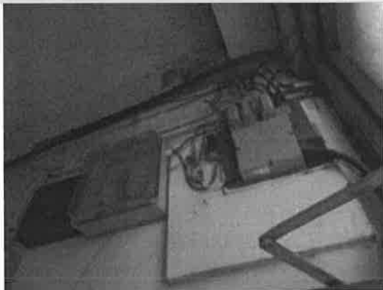
Exposed wiring in communal close
