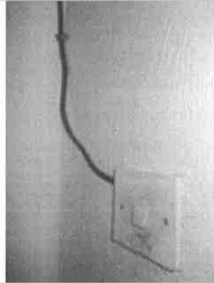
Light switch in back room - exposed wiring
