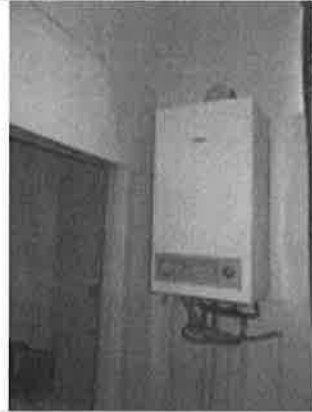
Boiler in back room
