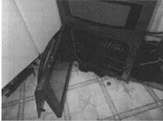
Kitchen in recess - cooker/defective oven door
