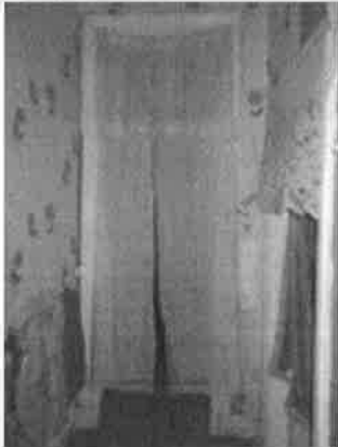
Hall - no door to living room
