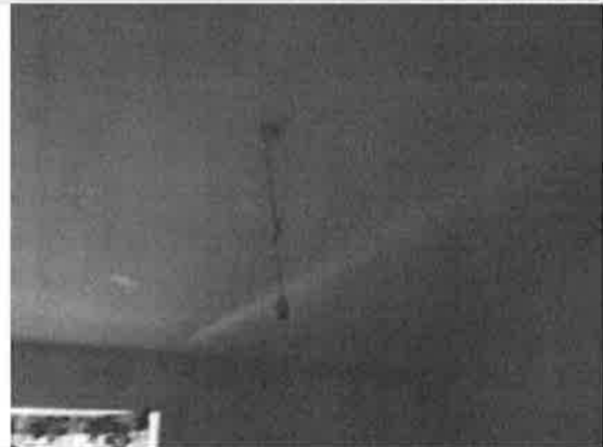
Light fitting in front living room
