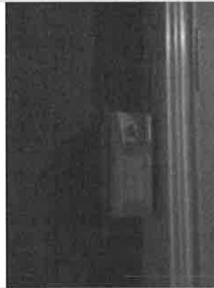
Door entry handset missing - Hall
