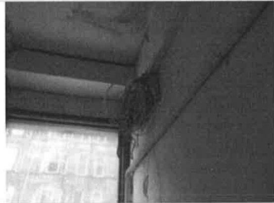
Exposed wiring in communal close
