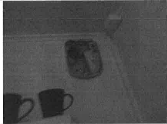
Extractor fan in Kitchen - missing cover
