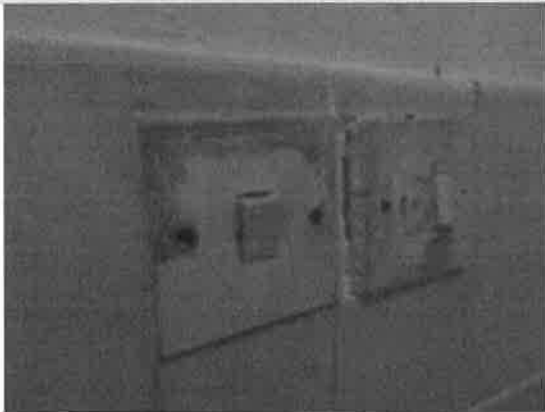
Switches in Kitchen
