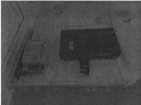
Fuse box in Hall
