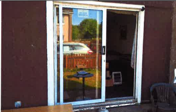
Patio Door. Ill fitting sliding door prone to come off sliding rail and fall out. Rotten timber at foot of door. The patio door unit requires repair/replacement.
