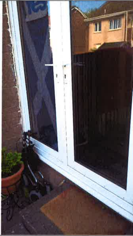
Rear door seals are ill fitting and door is very difficult to secure. The door unit requires to be repaired/replaced.
