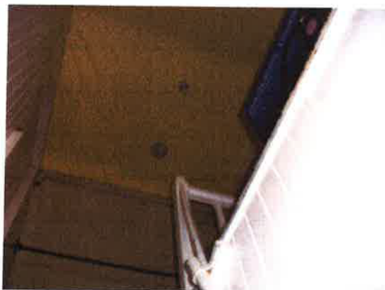
13 - Smoke detector - upper hall
