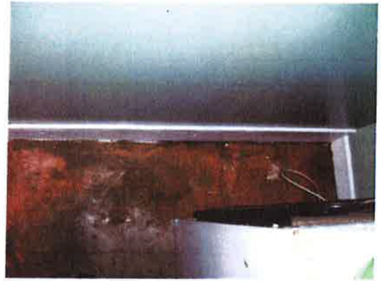
02 - Kitchen dampness floor at NE gable corner
