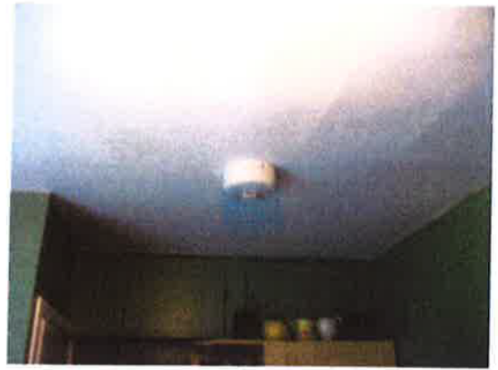
10 - Kitchen - Heat detector
