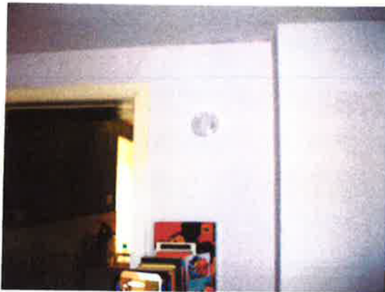
11 - Carbon monoxide detector - living room
