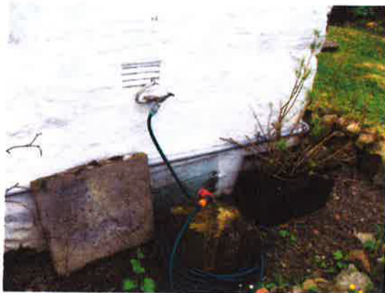
05 - Standpipe at NE gable
