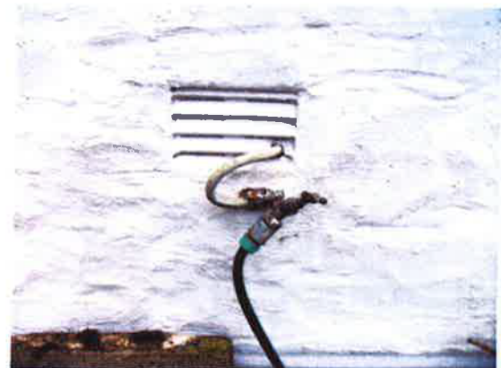
06 - Standpipe showing rubber supply pipe
