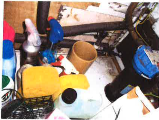
09 - Kitchen under sink showing supply pipe
