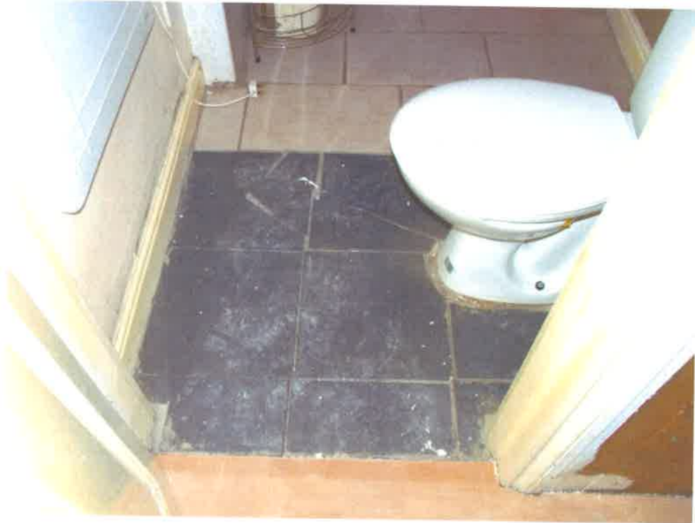
Damaged floor tiles in Shower Room
