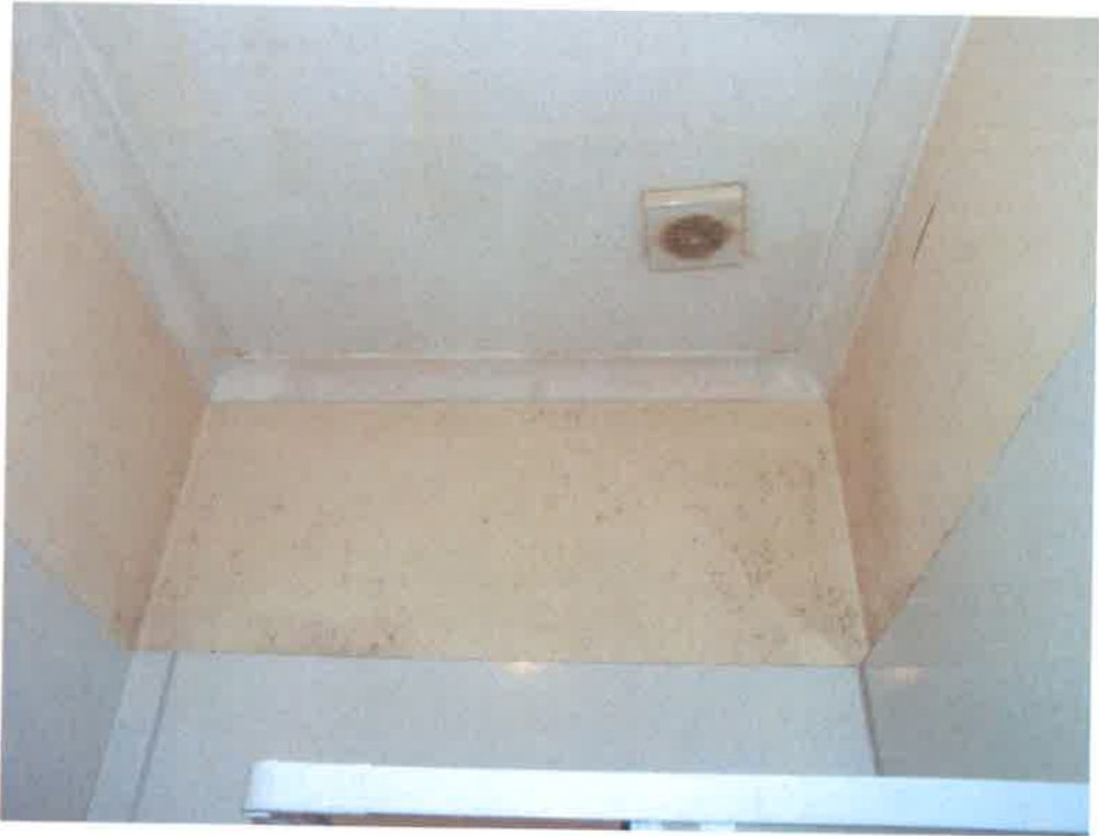
Condensation mould in Shower Room
