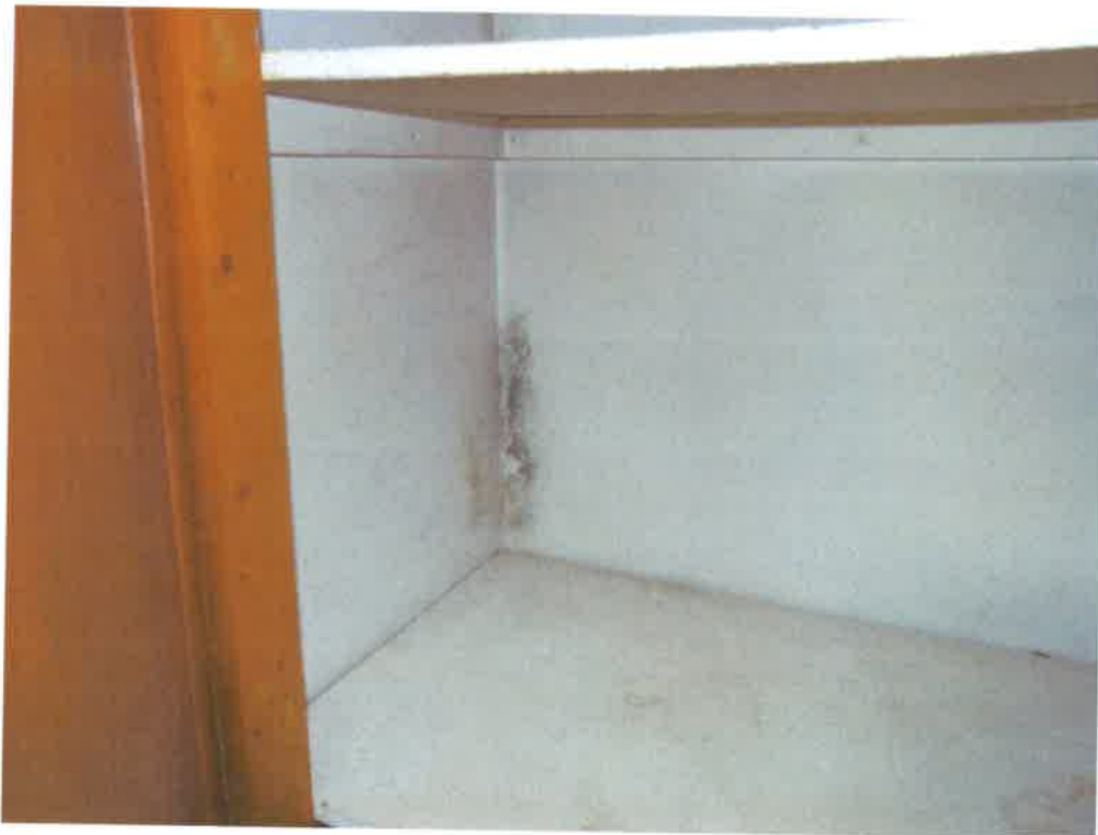
Condensation mould in Lounge cupboard
