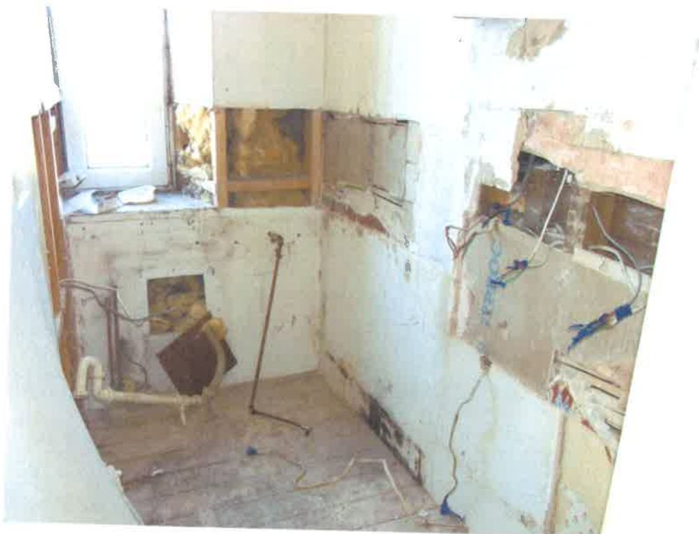
Condensation mould in Kitchen
