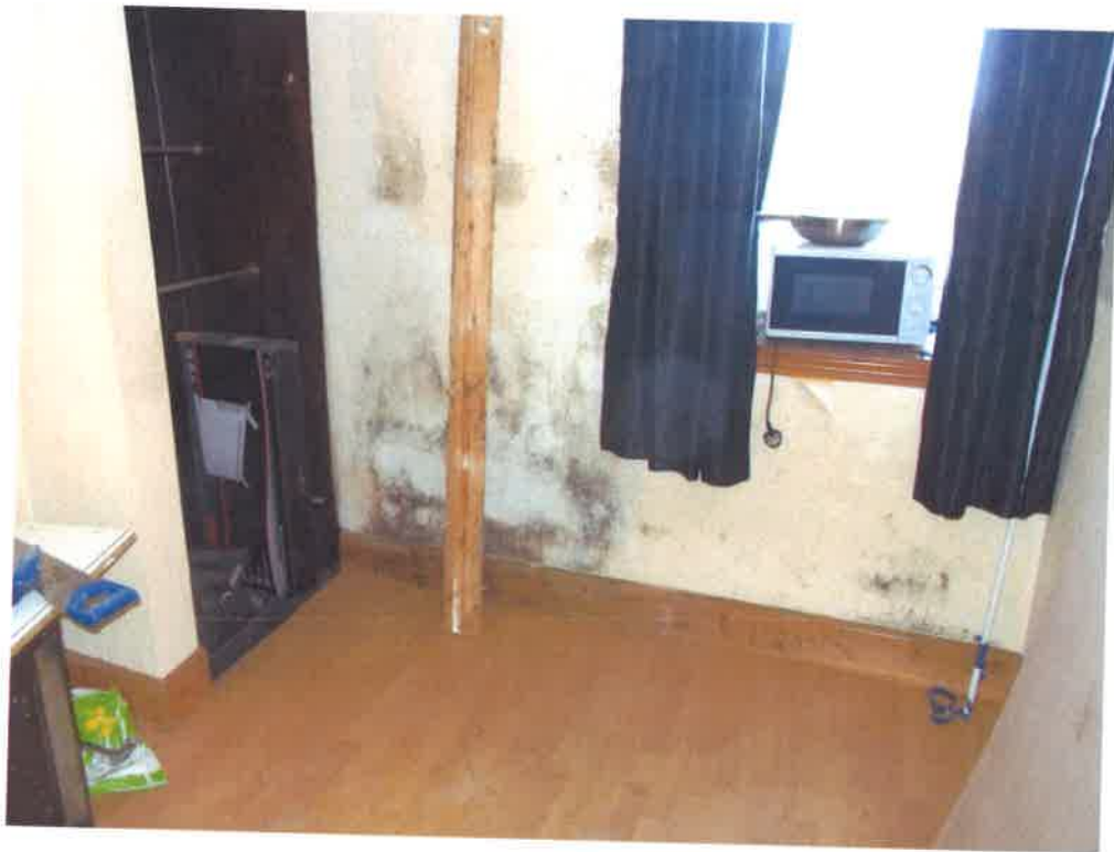
Condensation mould in Bedroom
