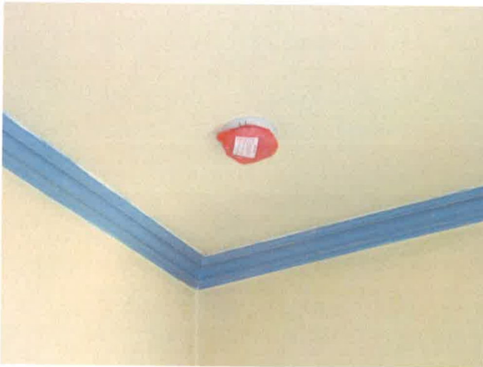
Lounge smoke detector
