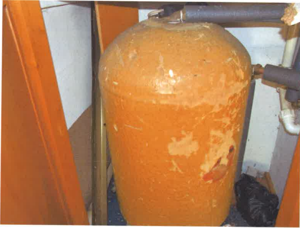
Hot water tank in Lounge cupboard
