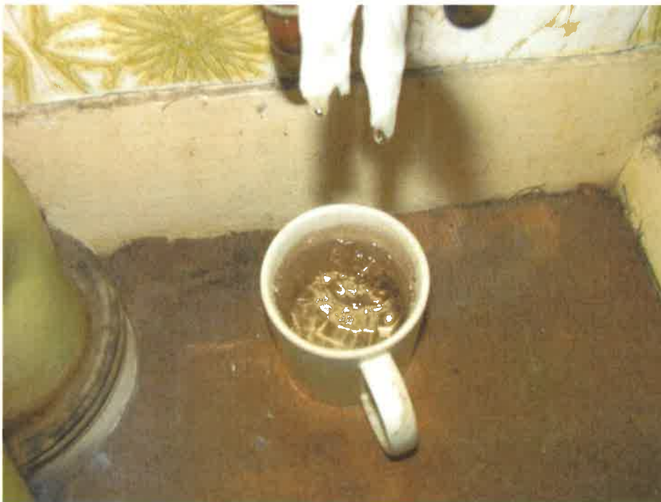
Leaking cistern/pipe work adjacent to W.C.
