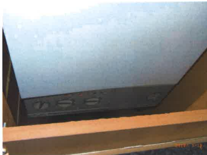
Central heating boiler
