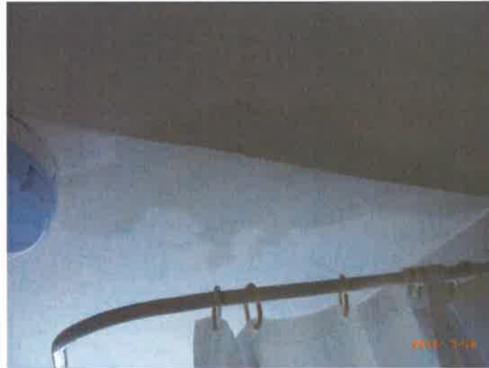
Damp staining on Bathroom ceiling
