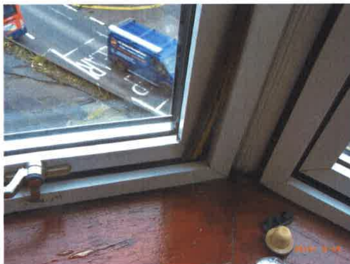
Loose seal at Lounge window
