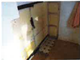
11. Missing Kitchen Units
