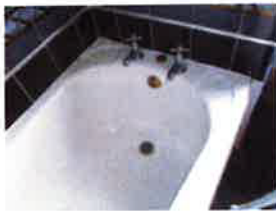
17. Loose Bath Waste
