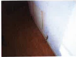
14. Missing Radiator Kitchen
