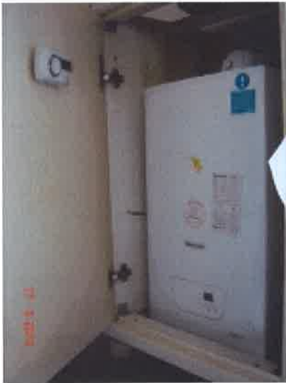
Gas boiler/CO detector
