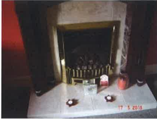
Living Room gas fire
