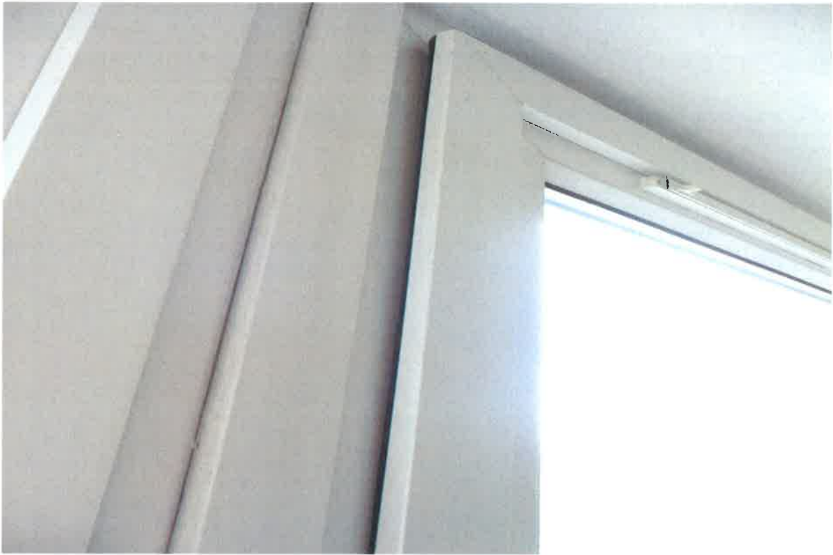
Bedroom 1 - Window in closed position showing gap to edge which admits draught
