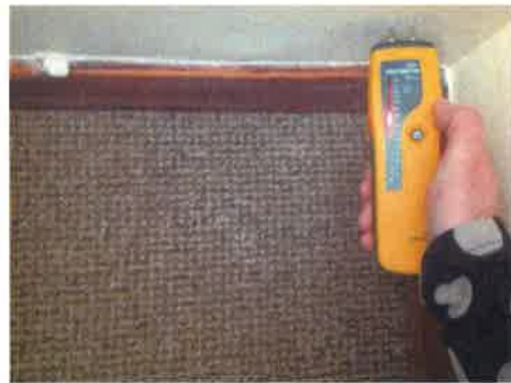
Bedroom – damp meter readings
