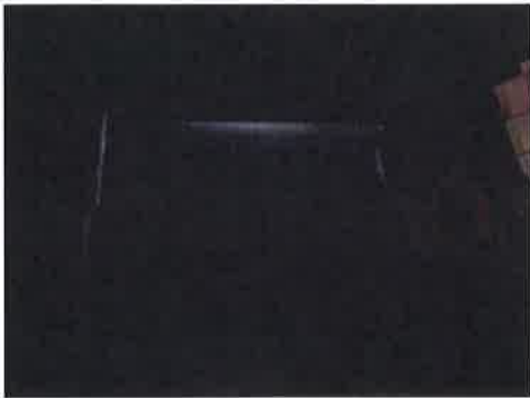
Front door – daylight showing through gap at bottom
