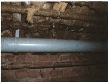
7. Leaking pipe - basement
