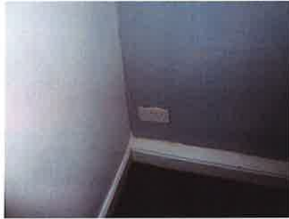
9. Bedroom Electrical Socket
