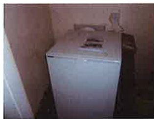
12. Oil-fired Central Heating Boiler
