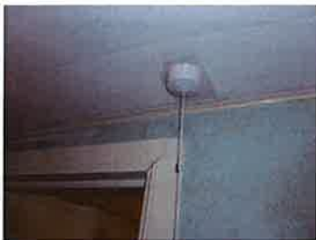
11. Bathroom Light Pull Switch
