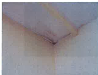
3. Mould at Living Room
