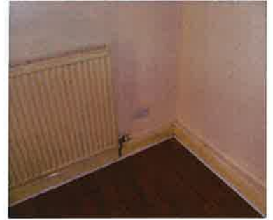
10. Bedroom Electrical Socket
