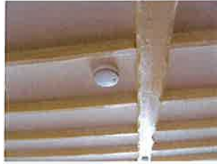
15. Hard Wired Smoke Detector Living Room
