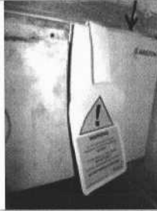
Kitchen - Boiler showing warning notice
