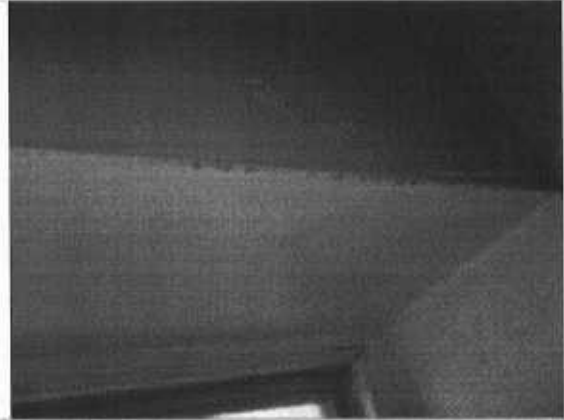
Main Bathroom - wall above window
