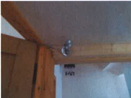
Light fitting to rear hall
