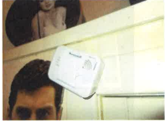
CO Alarm on door to boiler cupboard
