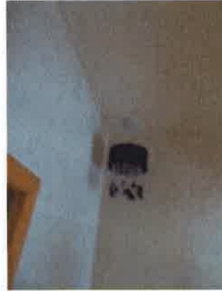
Light fitting to rear hall
