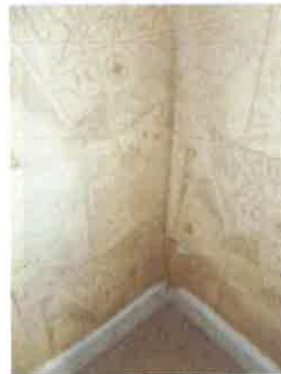
Son's Bedroom corner of rear single storey projection
