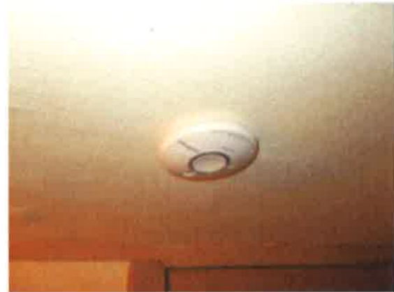
Smoke alarm - ceiling mounted - Hall
