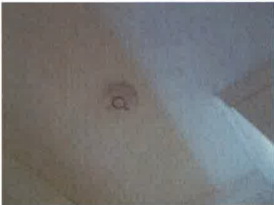
Smoke alarm ceiling mounted - Hall
