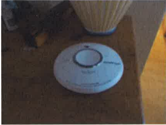
Smoke alarm not fixed- Hall
