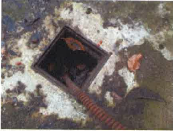
External drain to rear
