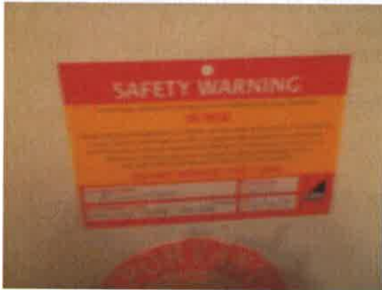
Safety Warning label on Boiler "At Risk"
