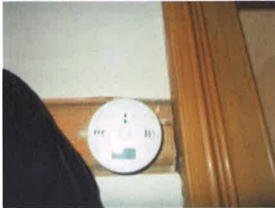
CO alarm on coat rack in Hall
