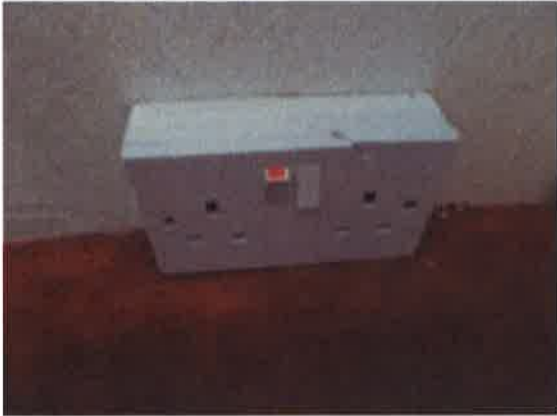
Cracked double socket (daughter's bedroom)
