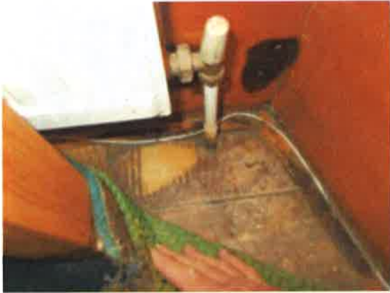
Kitchen - radiator and carpet (lifted to expose floorboards)
