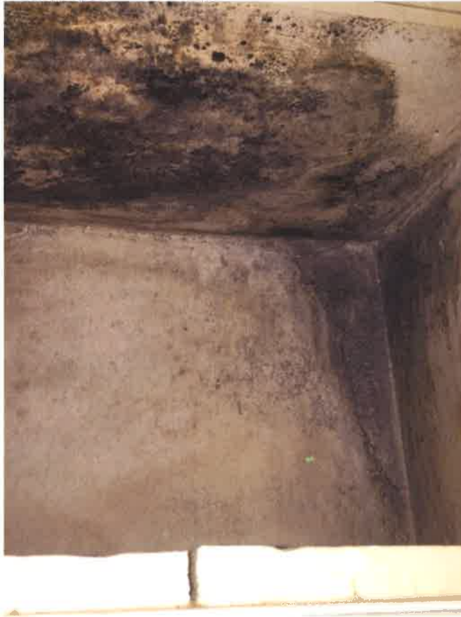
Photograph 4: Top of cupboard showing extensive black/grey mould walls and ceiling
