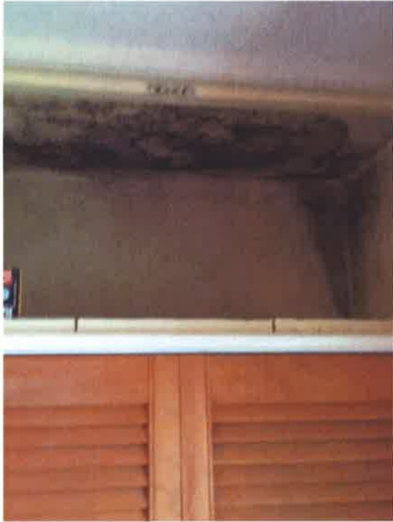
Photograph 5 : Cupboard ceiling showing damaged ceiling panel and black/grey mould
