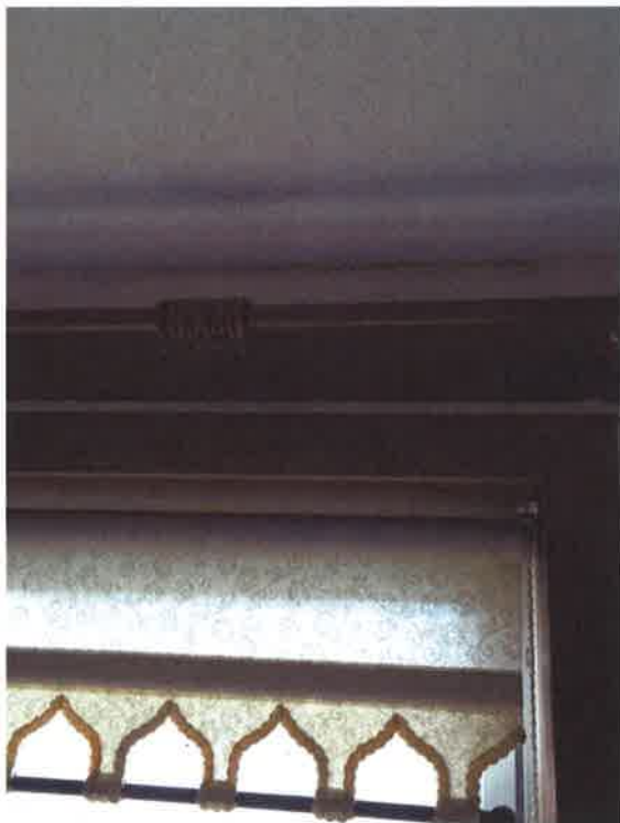
Photograph 6 : Showing black/grey mould above curtain rail at ceiling
