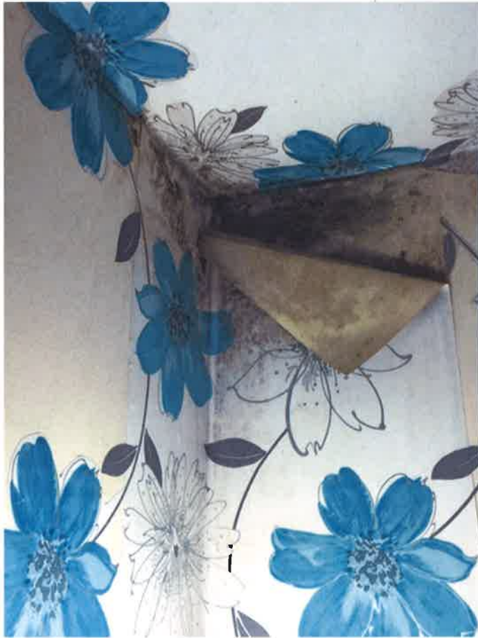
Photograph 3: Corner of room at ceiling showing black/grey mould on walls and wallpaper
