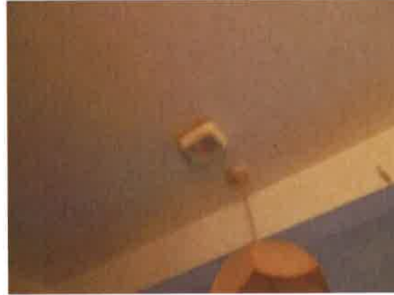
Smoke alarm in Hall
