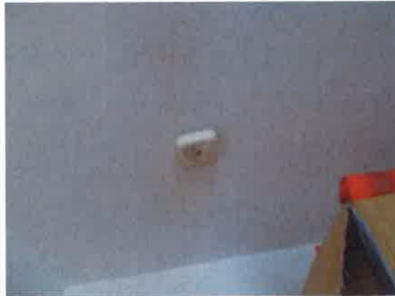
Smoke alarm in small front bedroom
