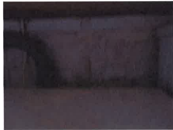
Kitchen - wall to rear of tumble dryer
