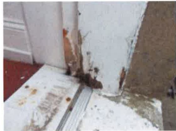
Rot to External door frame
