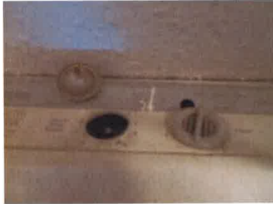
Defective control knob to electric heater in Living Room
