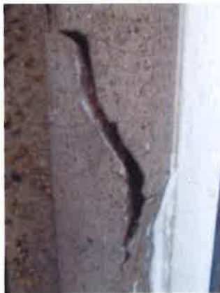
Crack to side of bathroom window to rear elevation
