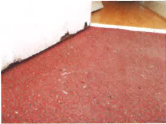
Rot to base of External door
