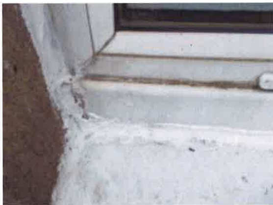
Sealant at Bathroom window - external
