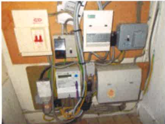
Fuse box in Hall
