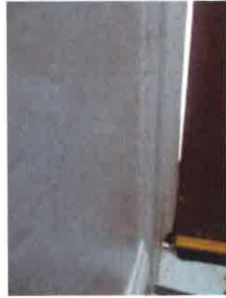
Gap at side of External door - view from entrance vestibule
