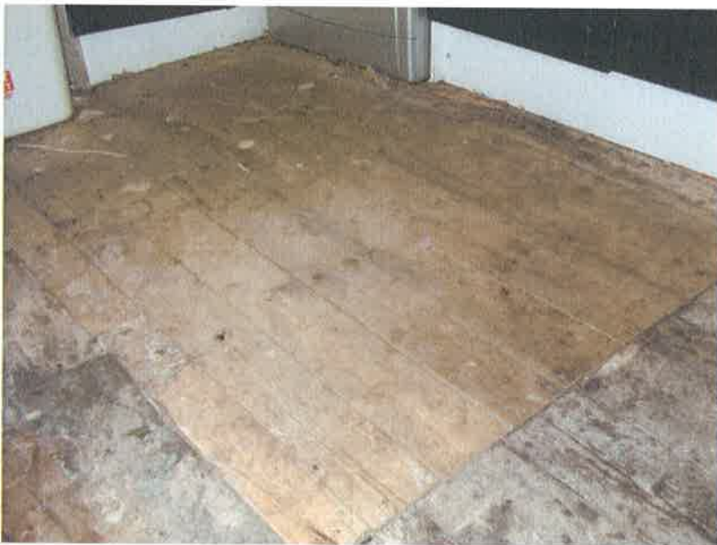
Kitchen Floor Timbers (and missing floor covering)
