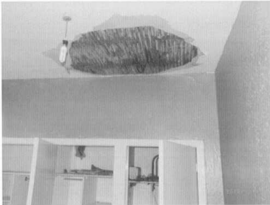
Damage to Bedroom ceiling
