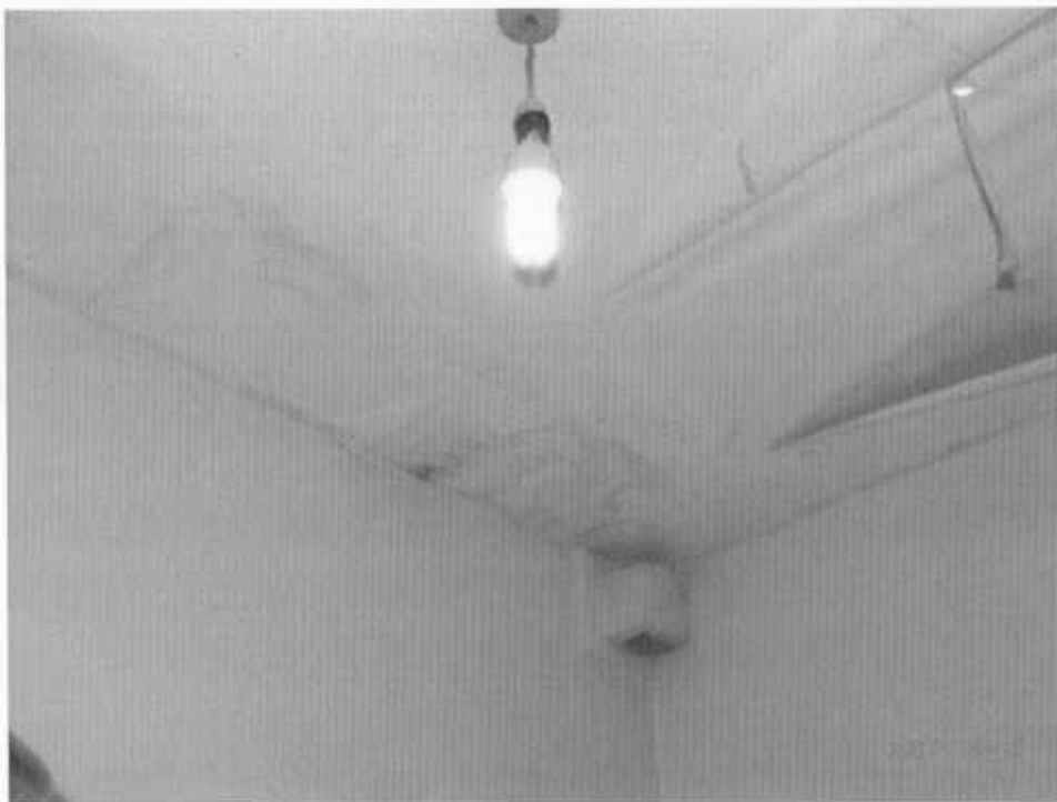
Damp staining/damaged plasterwork and decoration to Bathroom ceiling
