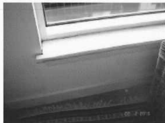
Loose Bedroom sill/plaster
