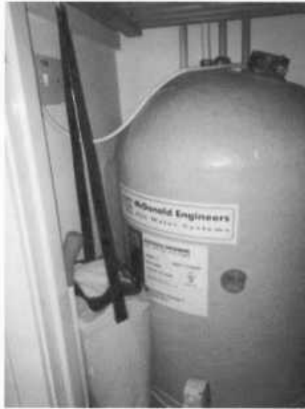
Immersion heater and hot water cylinder tank
