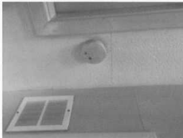
Inner hallway – battery operated smoke detector
