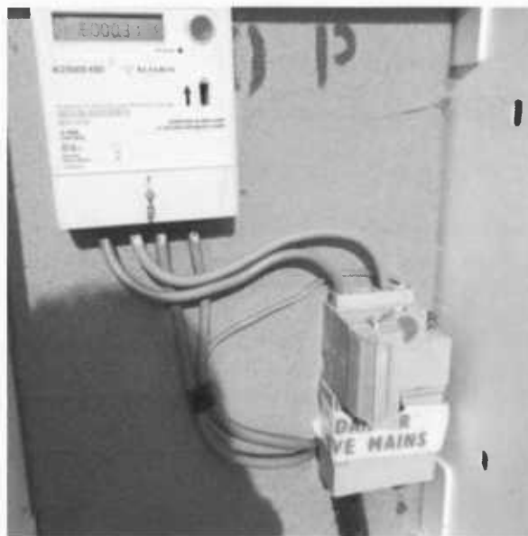
Meter cupboard – electric pre-payment meter
