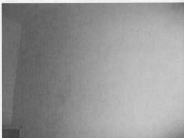
03- Wall showing dampness
