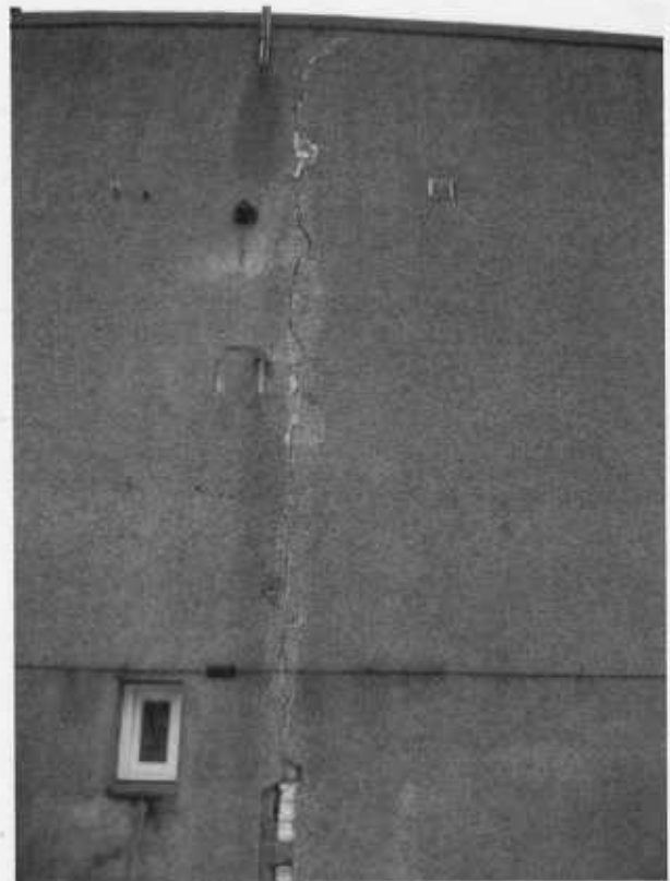
09 - Vertical crack at No 70A
