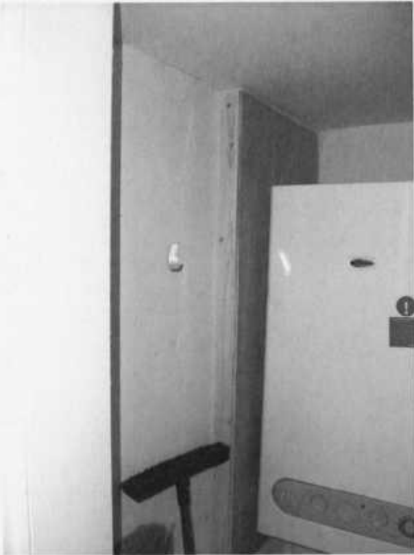
07 - Utility room – board fitted at boiler
