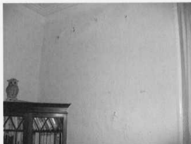
04- Wall showing bulging and loose plaster
