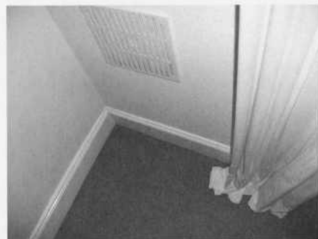
06- Dampness carpet (below vent)
