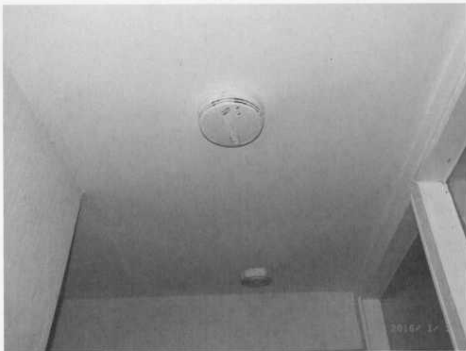
Hall smoke alarm
