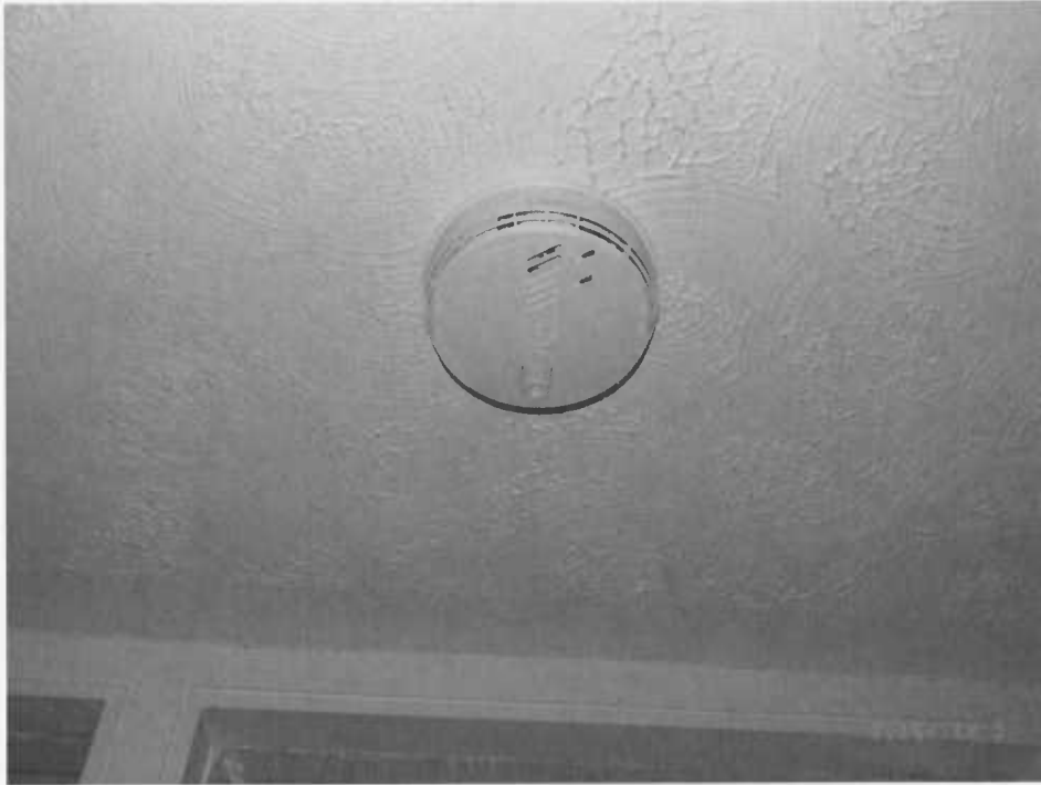
Lounge smoke alarm
