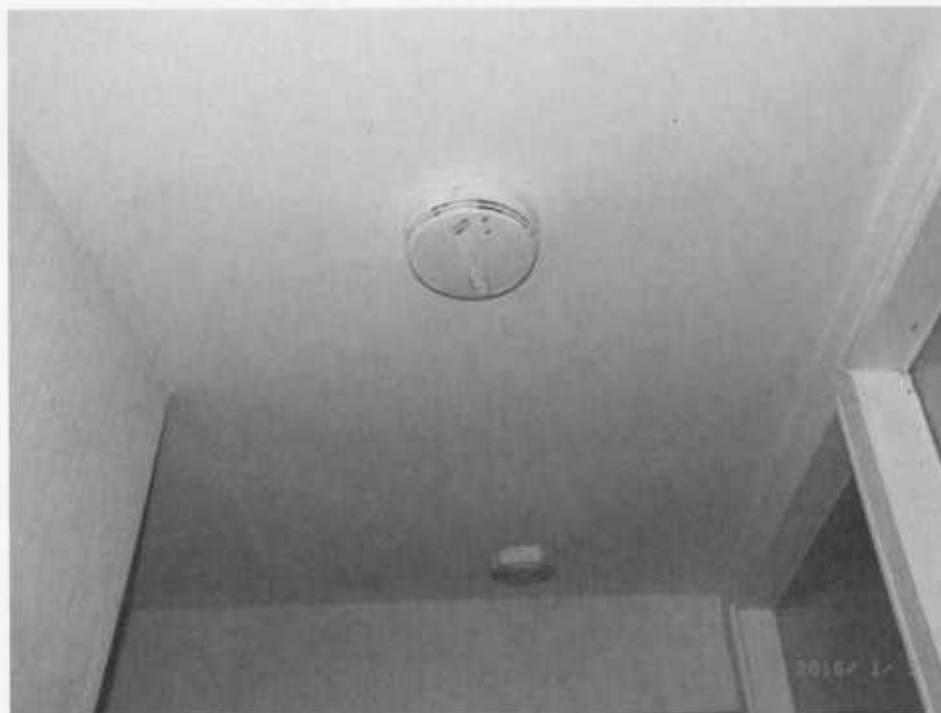
Hall smoke alarm
