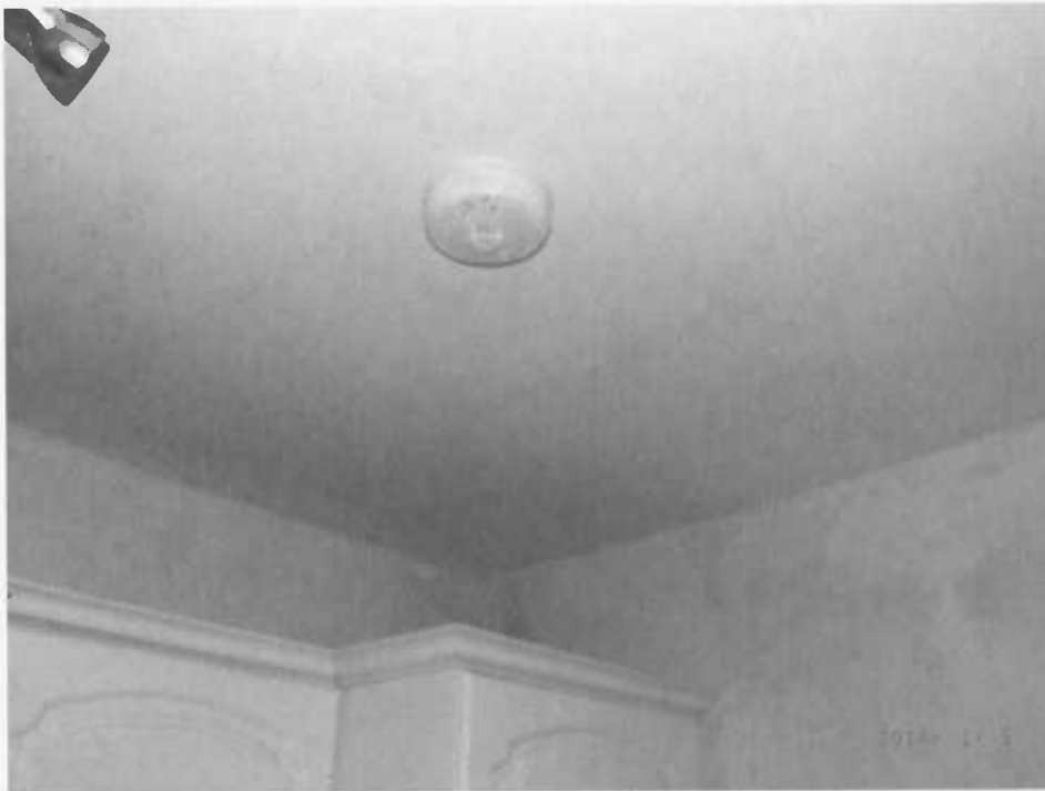
Kitchen smoke alarm
