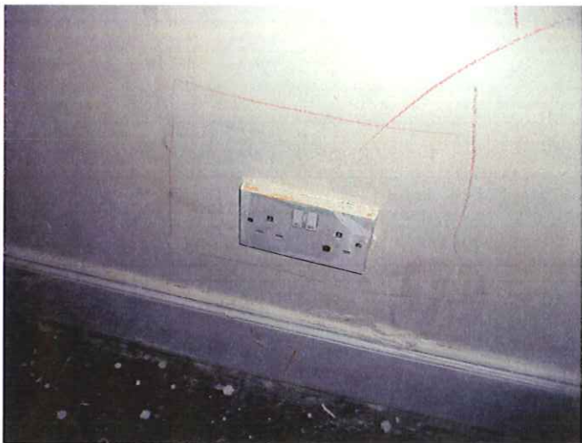
03 – Faulty socket in living room
