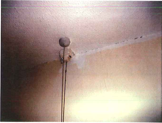
07 – Pull switch in bathroom
