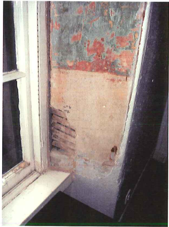
10 – Missing plaster at rear bedroom window
