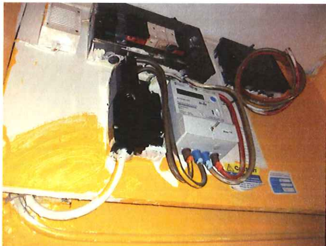
11 – Electric main board
