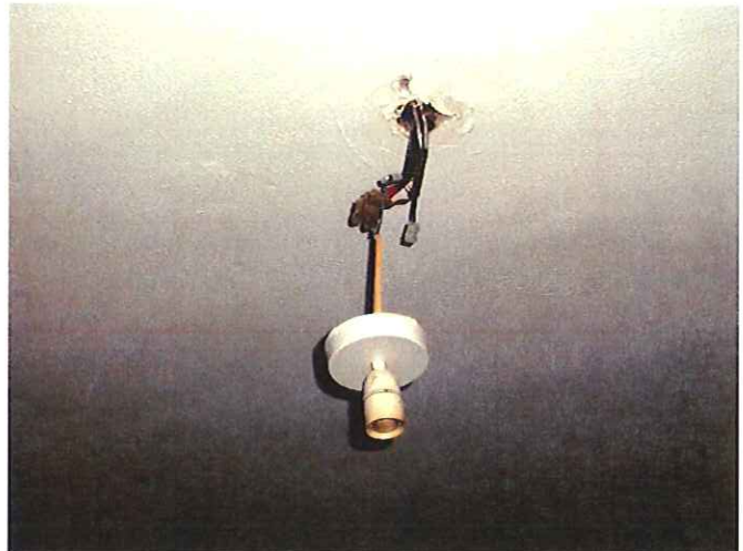
04 – Light fitting in living room
