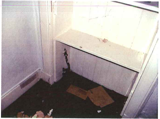
08 – Gas supply pipe in rear bedroom
