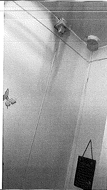
Shower switch does not work
