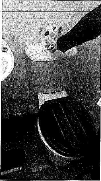
String used for flush on cistern
