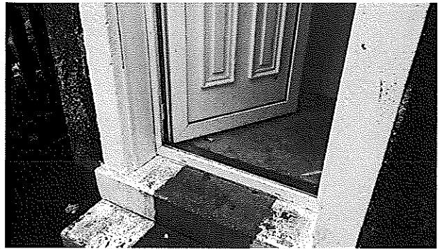
Poorly fitting front door
