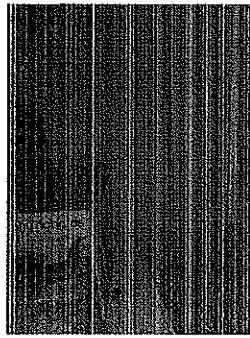
Damp wall at back door
