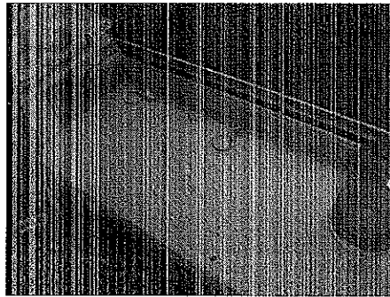
Water penetration living room window
