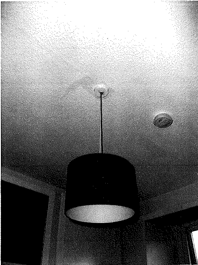
09 – Rear bedroom - Carbon Monoxide detector Boiler in lower cupboard, left of light
