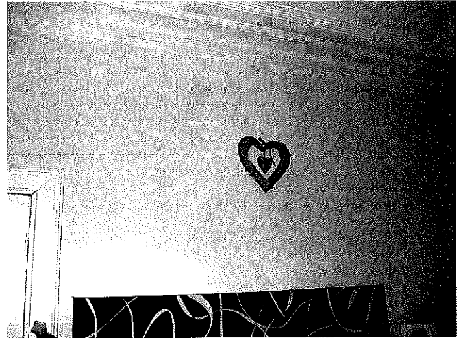
08 – Dampness - living room (chimney) wall
