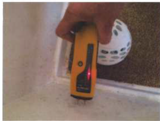
Bedroom – damp meter reading
