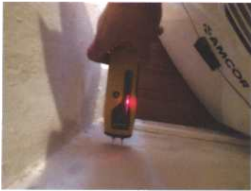
Living room - Damp meter reading
