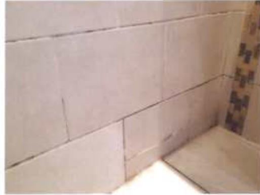
Bathroom – broken tile
