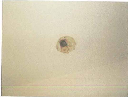
Living Room - smoke alarm
