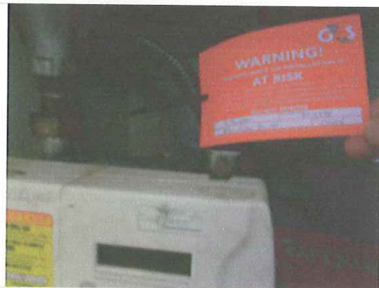
Kitchen - Gas Meter - warning label
