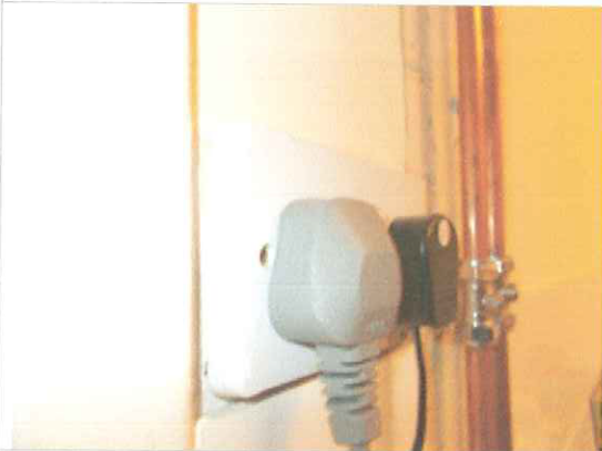
Kitchen - Loose double socket
