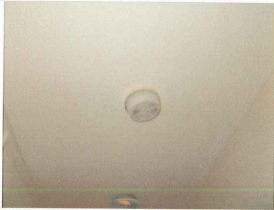
Hall - smoke alarm
