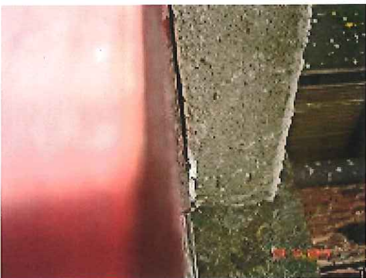
LR window-defective pointing
