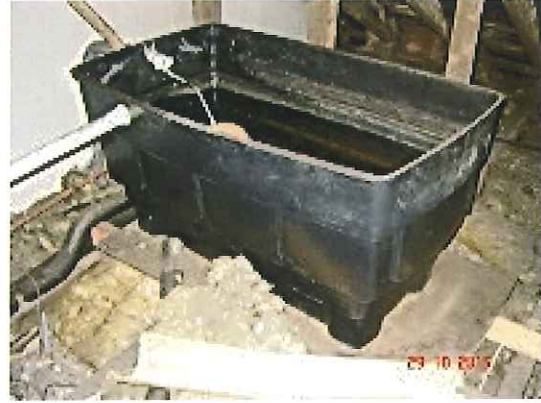
Attic – cold water tank
