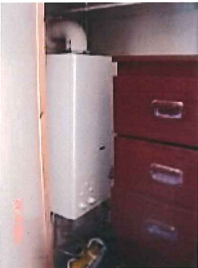
Central heating boiler
