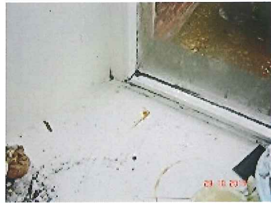
LR-damp stain on window sill
