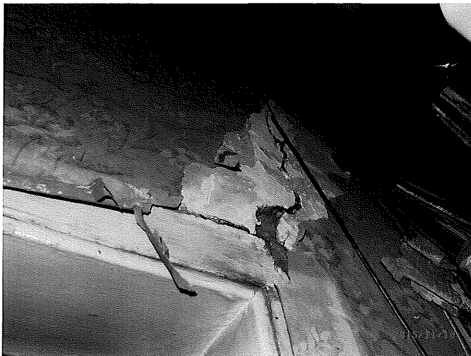
Crack in Lounge cupboard plasterwork
