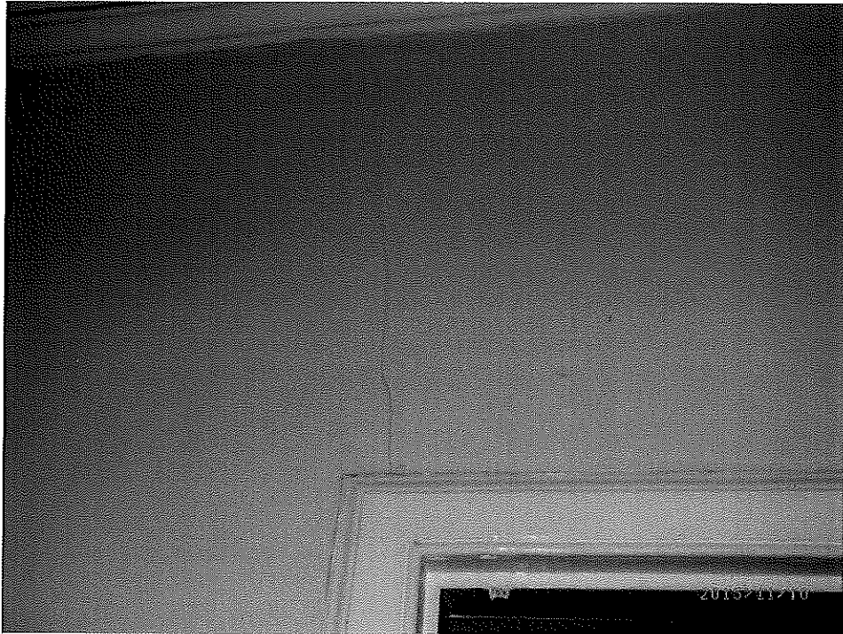
Crack in plasterwork above Kitchen door to Dining Room
