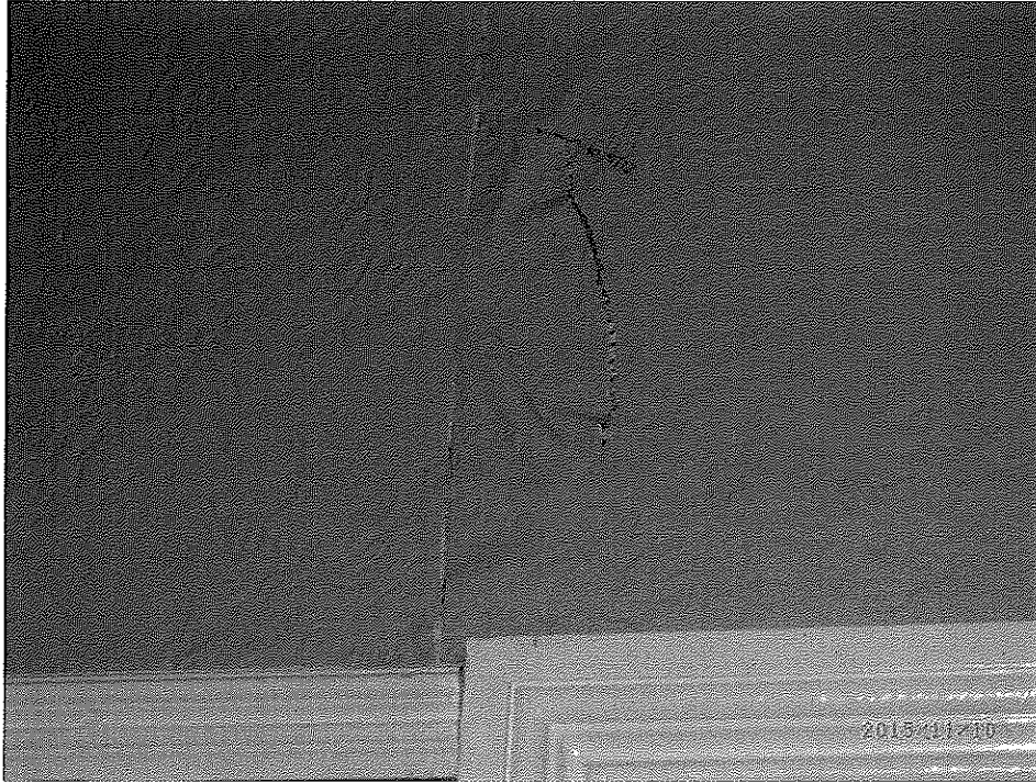
Crack in plasterwork in party wall between Lounge and Bedroom (mirrored adjacent)
