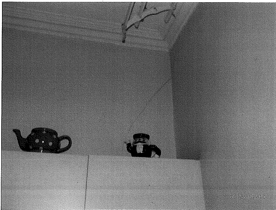
Crack in Kitchen party wall with Bathroom
