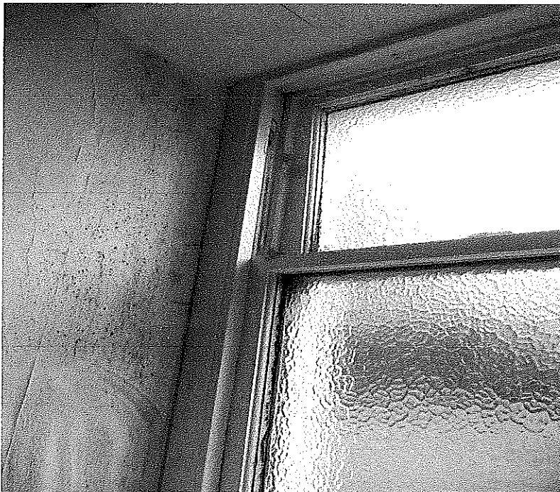
Bathroom window – painted shut
