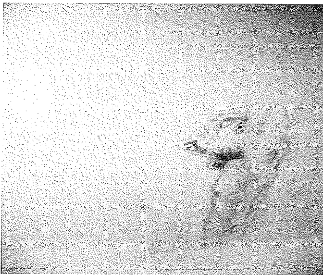
Kitchen ceiling showing leak from flat above
