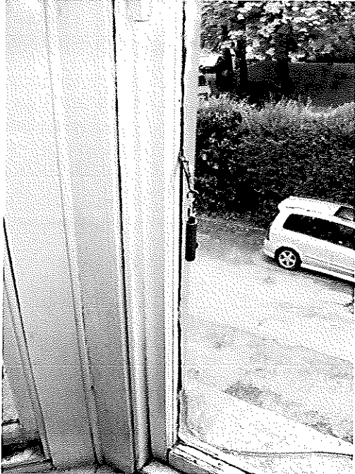
01 – bay window – gap at glass & frame
