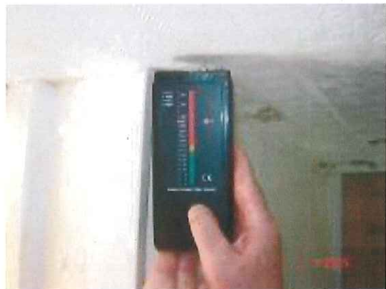
Damp reading-hall wall PHOTO 22
