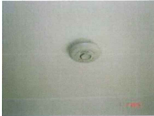
Ground floor hall - smoke alarm
