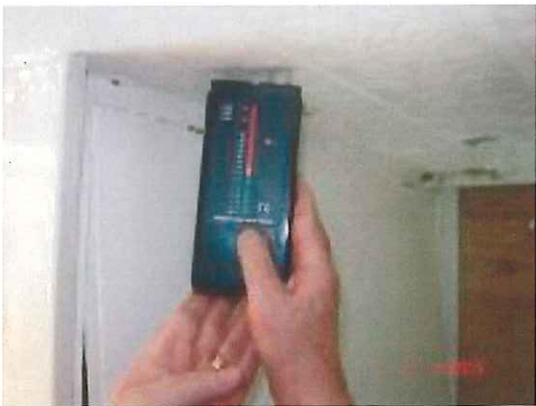
Damp reading-hall wall PHOTO 21
