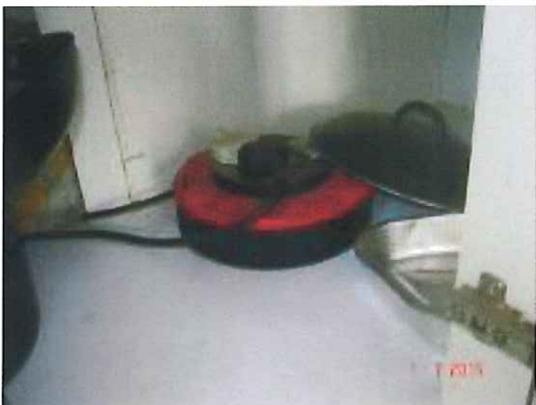
Cable extension in kitchen
