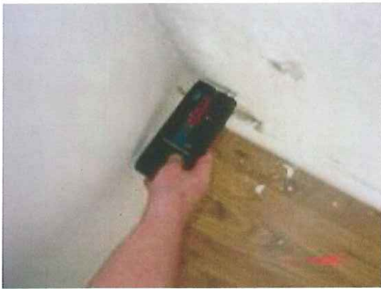
Damp reading-hall wall - PHOTO 19
