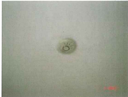
Upper floor landing – smoke alarm
