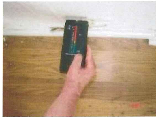
Damp reading-hall wall - PHOTO 20
